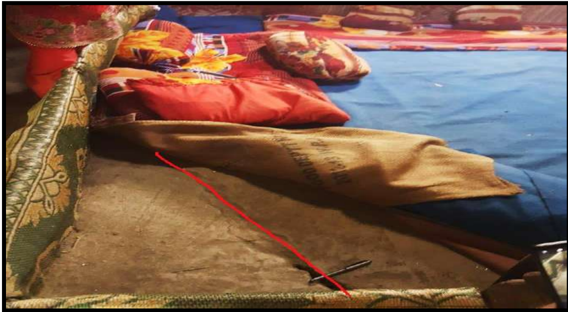
Figure 13: Cracks developed within the Houses
