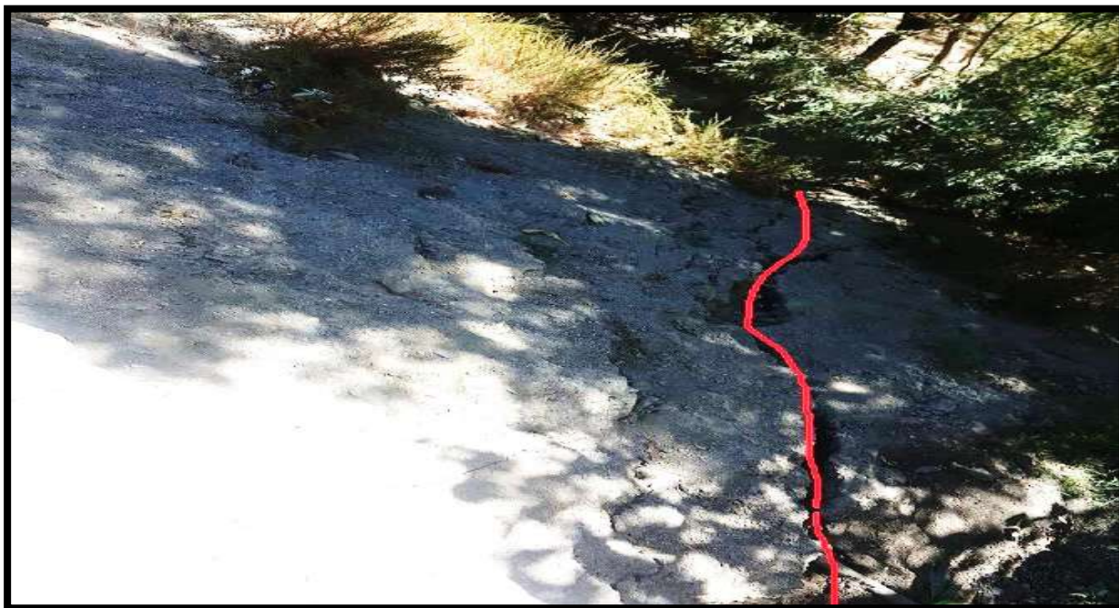
Figure 10: Deep Cracks touching bedrocks
